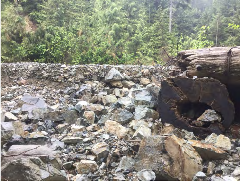
Downstream right bank fill has eroded away completely
